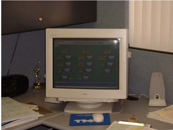
Computer screen that allows district personnel to monitor and control pumps throughout the district with the SCADA system.
