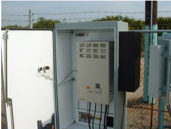
Enclosure and variable frequency drive panel at OCID.
