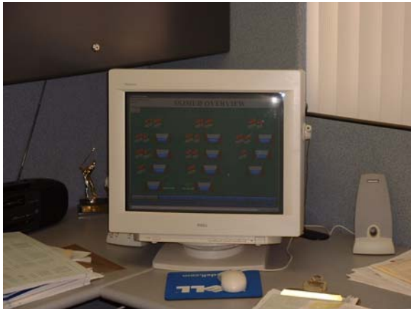
Computer screen that allows district personnel to monitor and control pumps throughout the district with the SCADA system.
