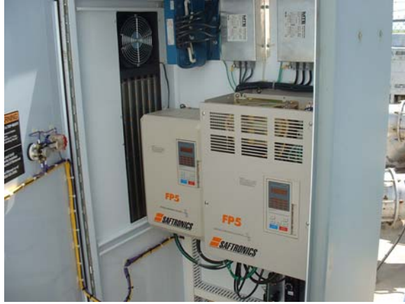
Two variable frequency drives at pump station C1. The station services two pipelines, with one VFD per pipeline.
