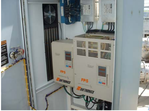
Two variable frequency drives at pump station C1. The station services two pipelines, with one VFD per pipeline.
