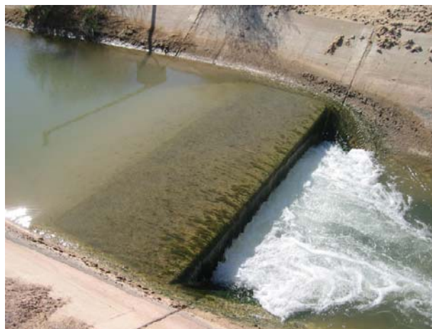
Figure 17. On-farm flume with maintenance issues, installed in a slip-form canal
