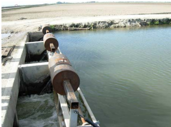
Figure 5. Three ITRC flap gates in parallel at San Luis Canal Company. These require no electricity, but must have a drop. There are hundreds of these throughout California.
