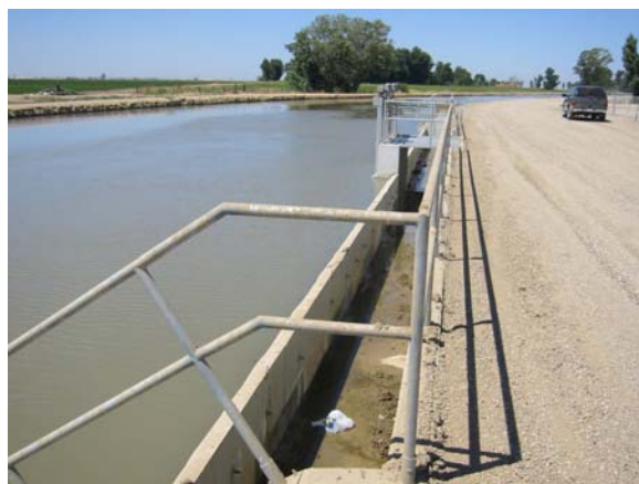
Figure 6. Special entrance to a 200 AF regulating reservoir at Central California ID. The sluice gates in the center are automated to open if the water level gets too high. Pumps at the upper right hand side (not seen) empty the reservoir if the water level in the canal gets too low. The long walls are for emergency spill into the reservoir.
