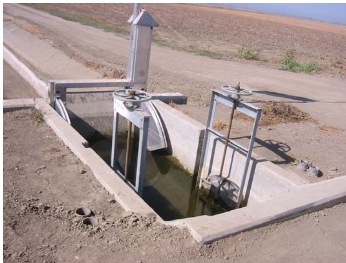
Figure 2. Example of an automated flow control turnout, with two adjacent manual turnouts
