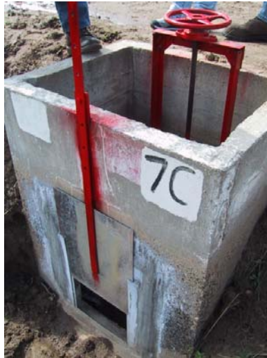
Figure 16. CHO at Alta ID. The orifice (on the canal, upstream side) is a standardized rectangle with an adjustable, bolt-secured opening. The downstream gate with the round handle is used to adjust the flow rate to the target.
