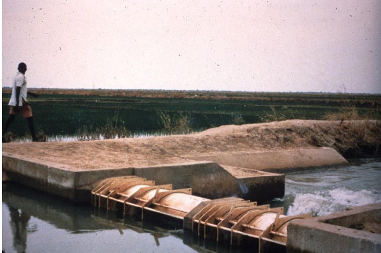
Figure 1. Baffle gates in Africa. Old, inappropriate technology for California.
