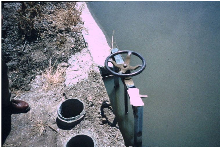
Figure 15. A classic metergate installation. The two round holes are stilling wells to measure the water level in the canal, and downstream of the gate. The gate is in the closed position in this photo (the stem is down).
