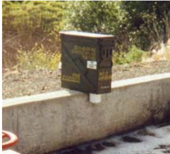
Photo 5. Field installation of portable water level monitoring package using an ultrasonic sensor. The installation is using the Milltronics Probe ultrasonic sensor and the ACR OWL datalogger.
