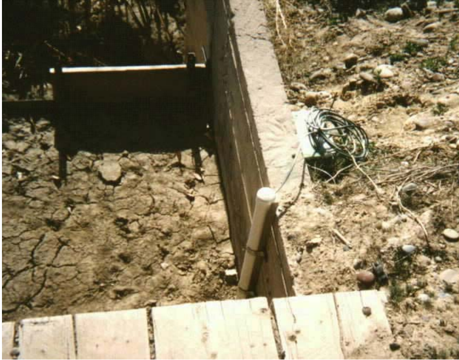
Photo 3. Field installation of portable water level monitoring package. The installation is using the Druck pressure transducer and the ACR OWL datalogger.
