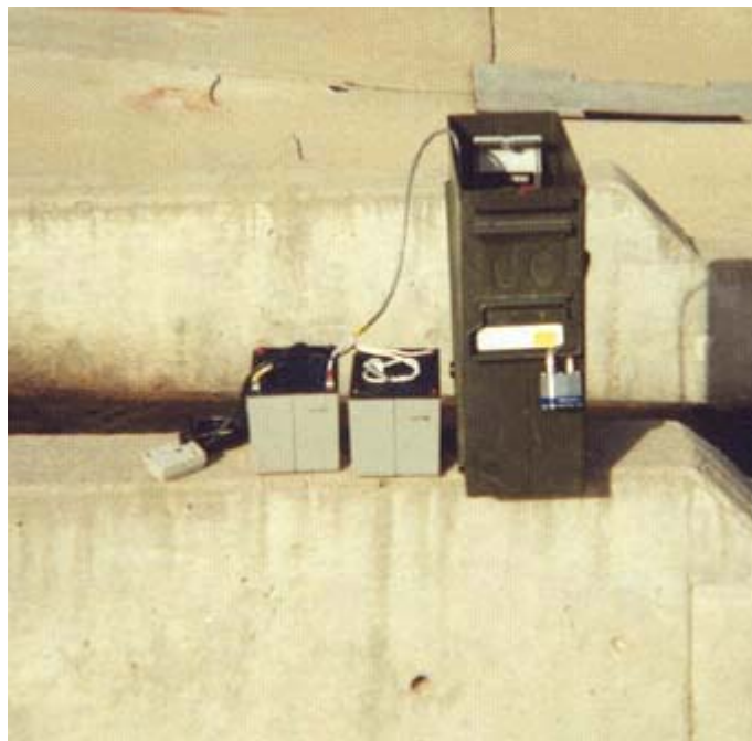
Photo 6. View inside the ammo box using the Milltronics Probe ultrasonic sensor and the ACR OWL datalogger. Note the size of the ammo box is 5.5" x 14" x 14". Also, 2 batteries are required for the installation because the Milltronics Probe requires more than 12 volts. Foam rubber was used to prevent the batteries from moving around inside the ammo box.
