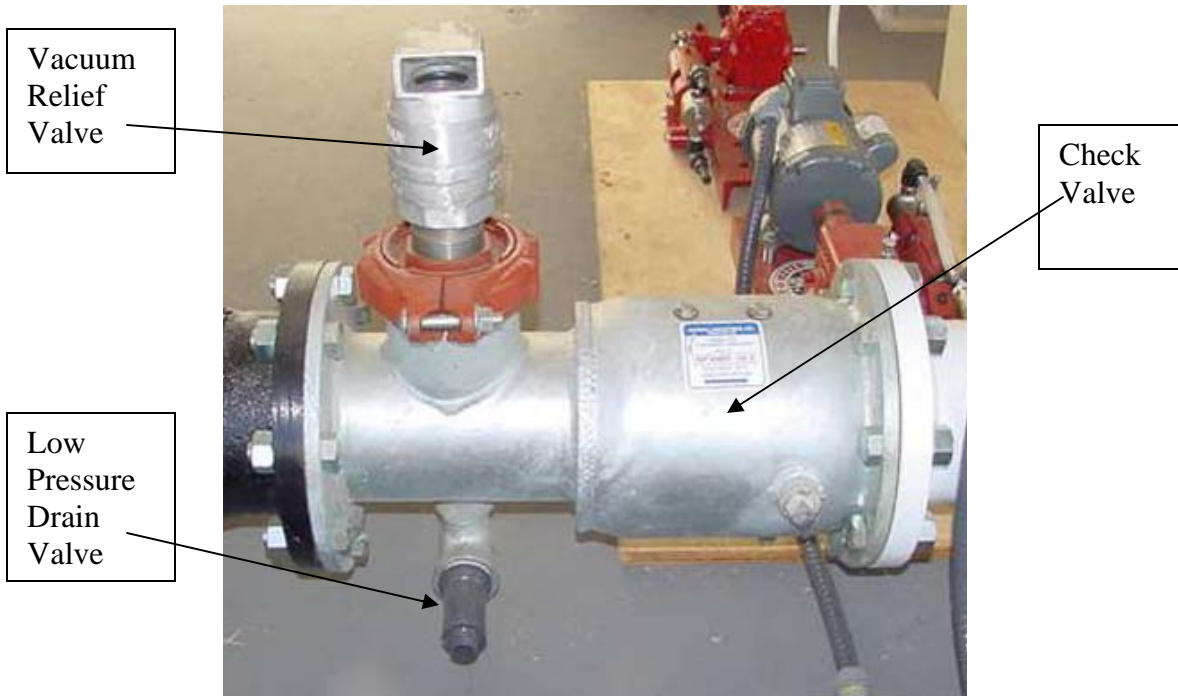
Figure 1: “Chemigation valve” (mainline check valve, vacuum relief valve, and low pressure drain)
