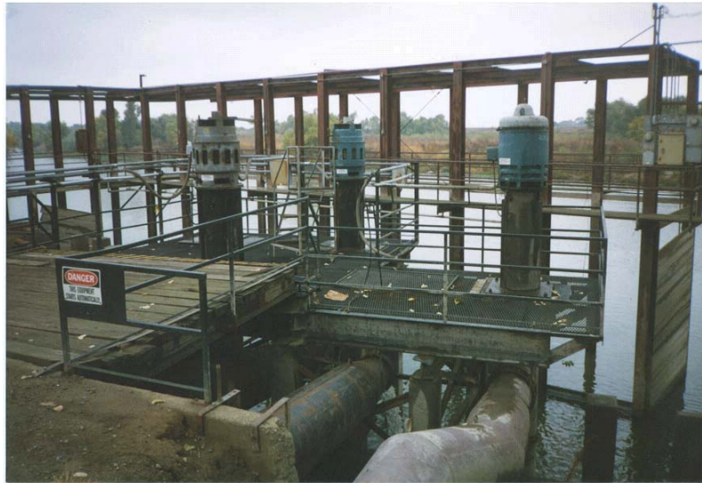
Figure 1. San Joaquin River Main Pumping Plant Showing 3 of 5 Pumps.
