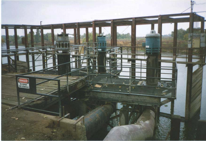
Figure 1. San Joaquin River Main Pumping Plant Showing 3 of 5 Pumps.
