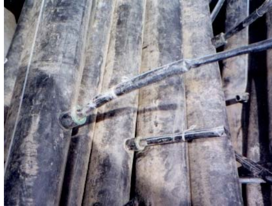
Figure 3. Manifold connection with punched socket fitting, a short section of polyethylene hose and wire ties to the tape.
