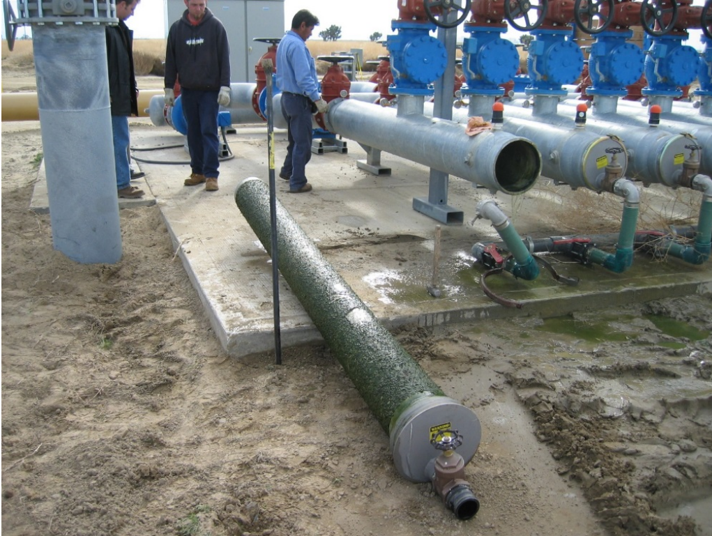
Figure 1. Typical horizontal cylindrical filter with a coarse, perforated stainless steel screen, typically used for sprinkler applications. Algae that passed through the screen can be seen on the downstream side of the screen. The complete screen has been removed from the filter housing. A 4" flush-through (not backflush) valve and hose manifold can be seen for each cylinder.
