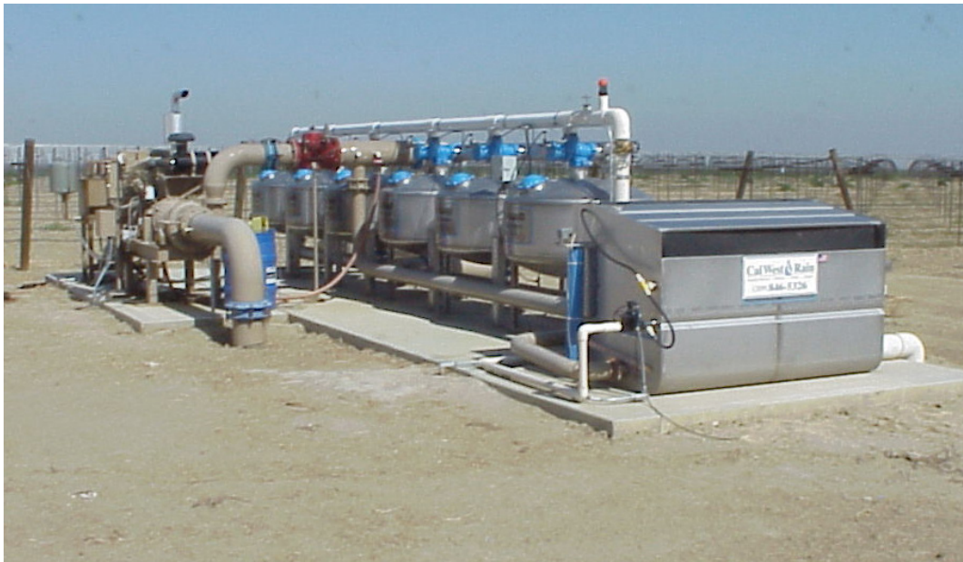
Figure 4. A media tank filtration system that uses a small commercial (FV&C) overflow screen to clean the backflush water before recycling it
