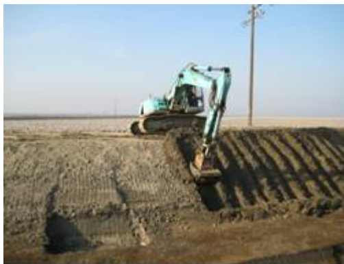
Figure 7. Compacting the canal banks on the James ID main canal with an MBW vibratory roller
