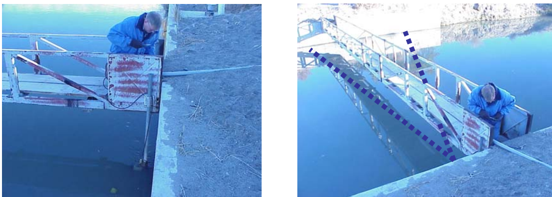
Figure 4. SonTek/YSI Argonaut SL installed in a canal
