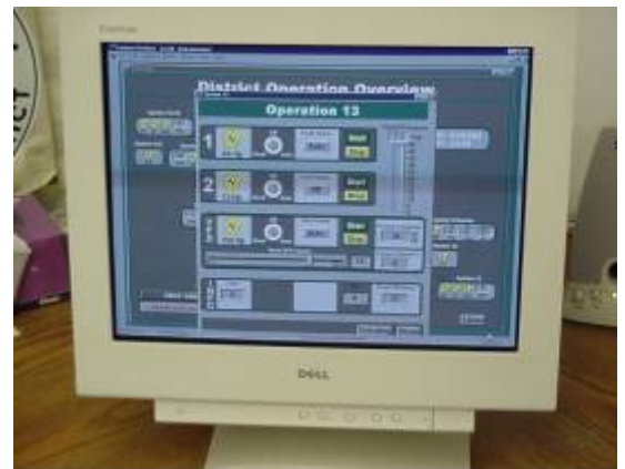
Figure 1. OCID SCADA screen in the district office.
