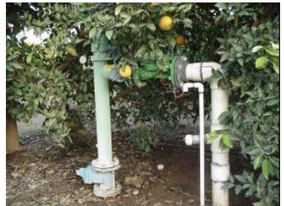
Figure 3. Automatic valve on a farmer turnout to shutoff deliveries before 12 pm and turn them back on after 6 pm.
