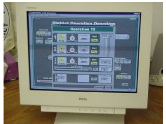
Figure 1. OCID SCADA screen in the district office.
