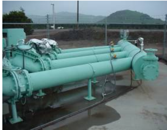
Figure 2. Pump station discharge outlet with new flow meters (yellow).
