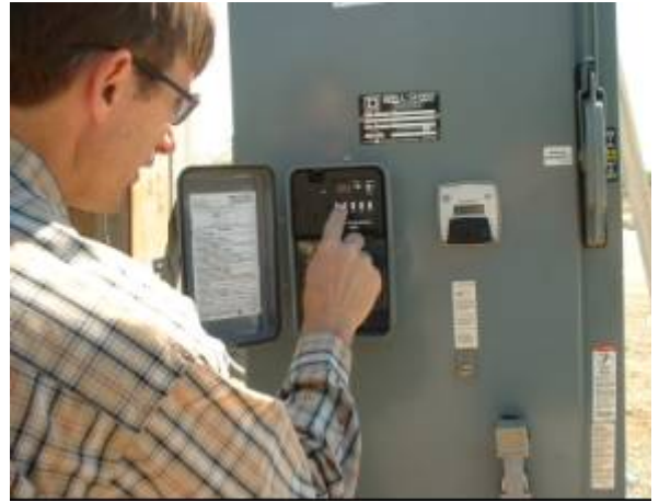
Figure 2. Clock timer used to automatically shut a groundwater well off before 12pm and turn it back on after 6pm every weekday during the peak season.
